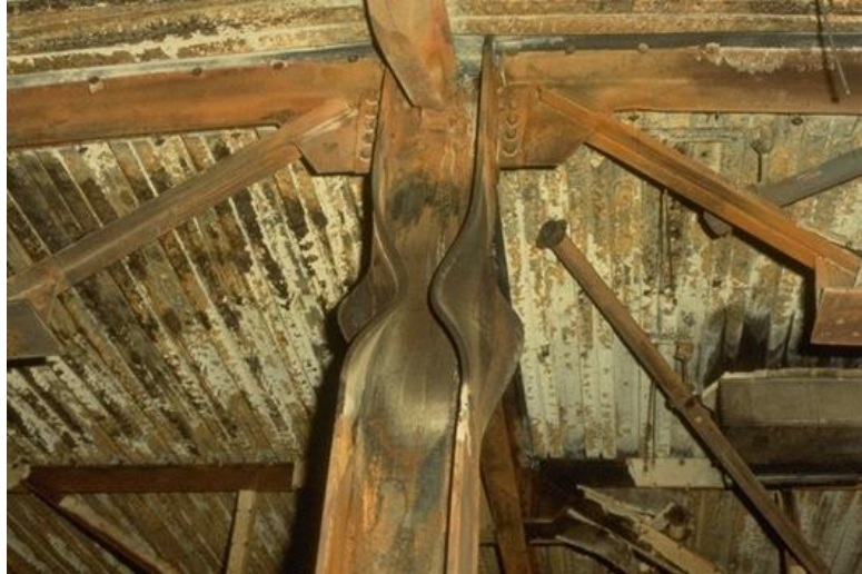
Figure 6: Deformed unprotected column in the Broadgate fire. Repairs were completed in 30 days
