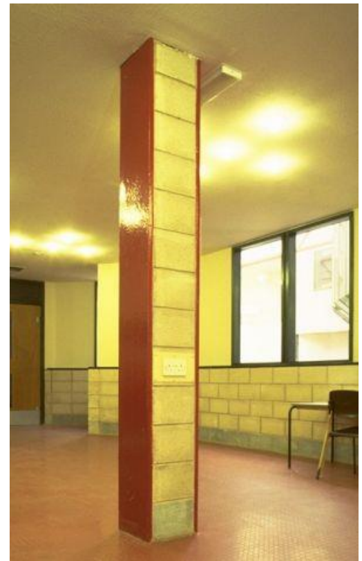
Figure 3: Columns, in-filled with blockwork between the flanges can achieve 30 mins fire resistance without applied protection
