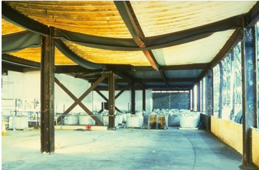
Figure 8: Deformed but stable structure after a fire in the Cardington eight storey building. No collapse occurred even though unprotected beams reached temperatures up to 1100°C.
