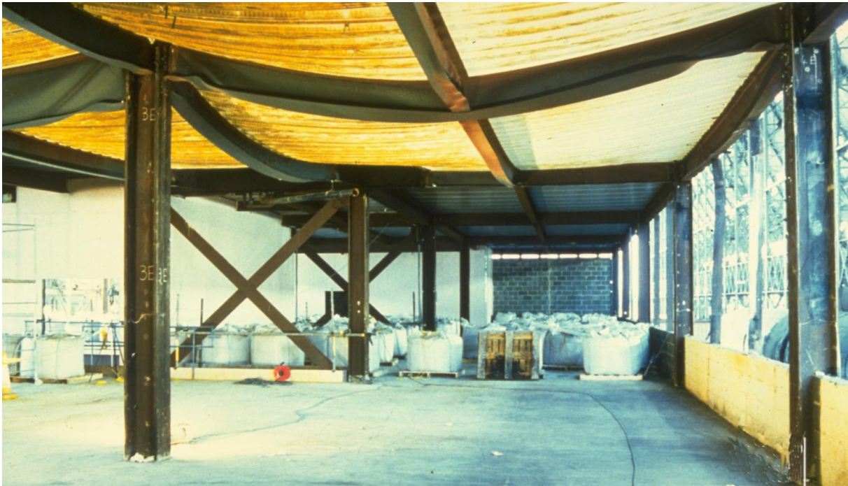
Figure 3: Deformed but stable structure after a fire in the Cardington eight storey building. No collapse occurred even though unprotected beams reached temperatures up to 1100°C
